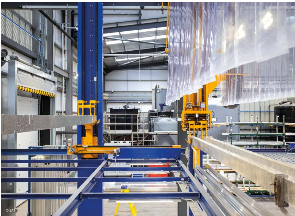
SAT designed an extra crane with a special design, operating at a higher level than the other bridge cranes, to eliminate the drop of productivity due to the return in counter-flow of the empty bars along the tanks line.
