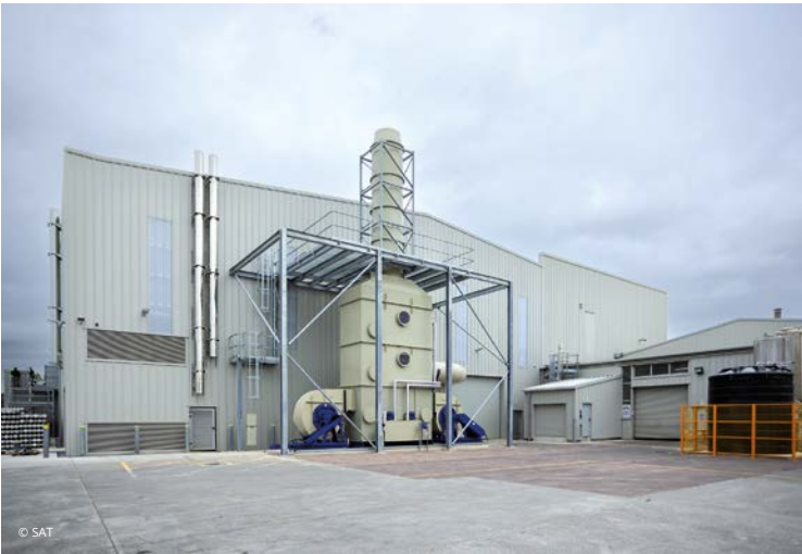
The air purification system.
